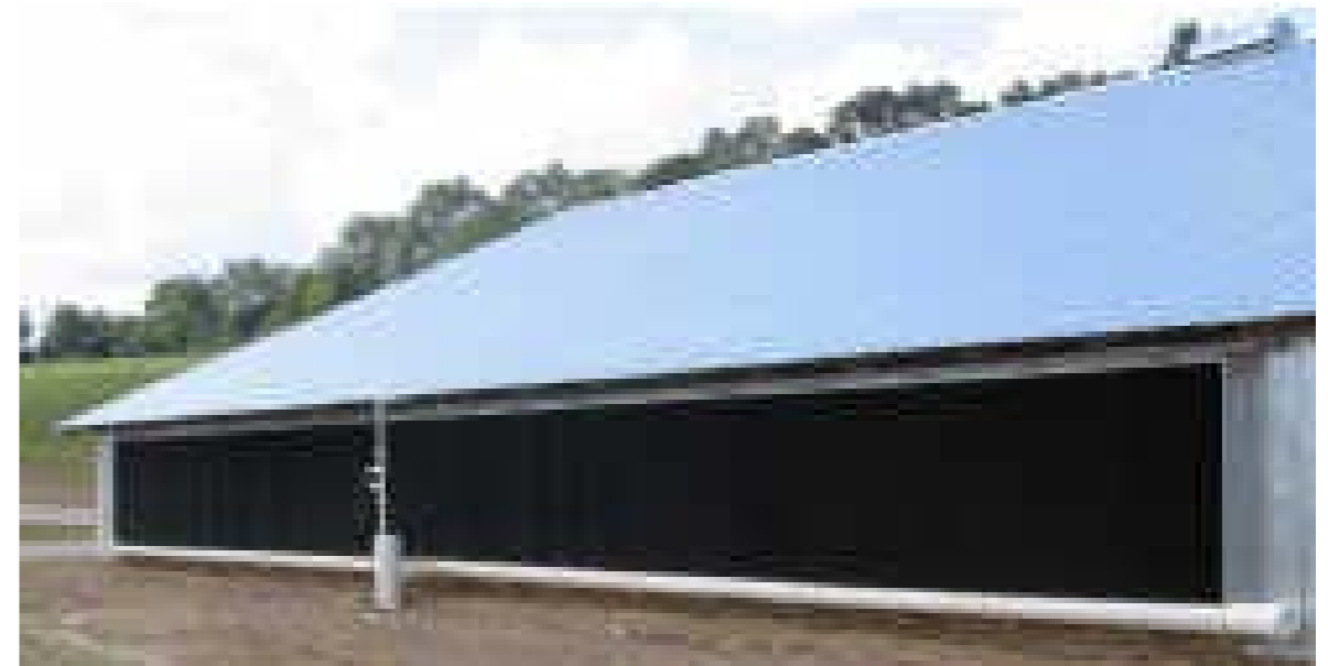
Recirculating Evaporative Cooling System
