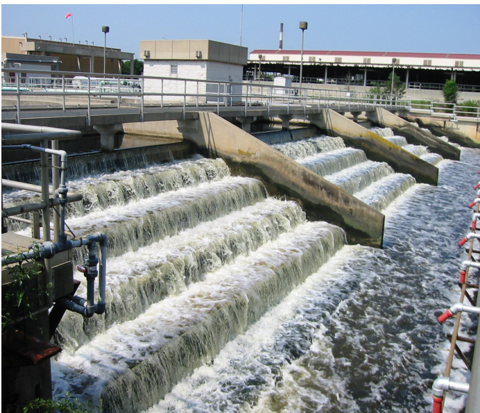
Using highly treated effluent from wastewater treatment plants (pictured) is called water reuse, water recycling, or reclaimed water. Photo by Dr. Rachel Rosenberg Goldstein.
