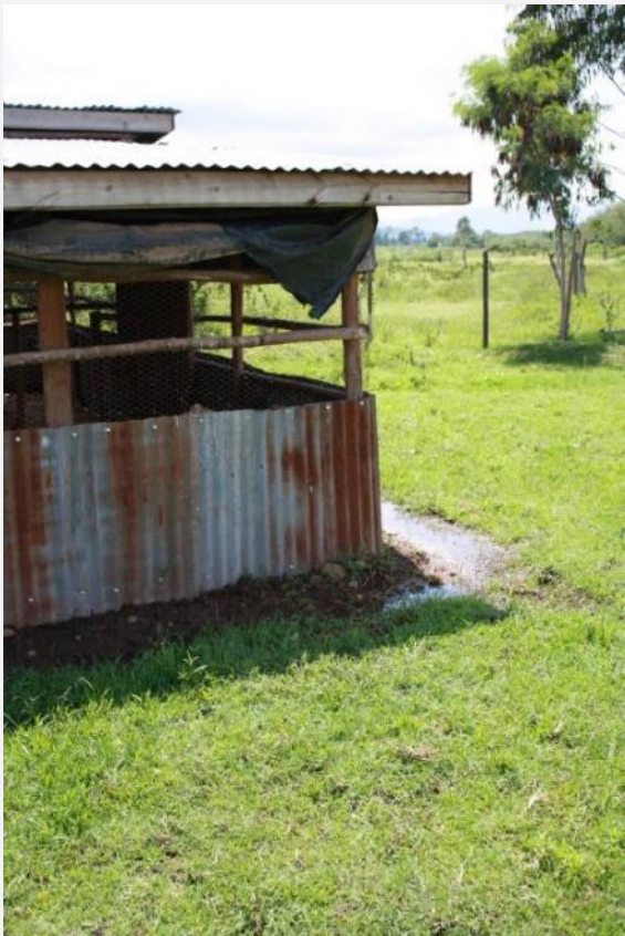
Poor storm water drainage
