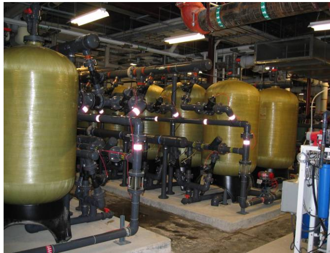
Hatchery filtration bank
