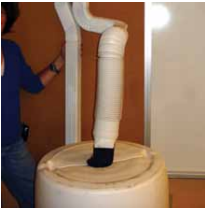
Downspout connection using flexible extender
