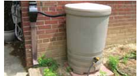
Rain barrel using in-line overflow adapter
