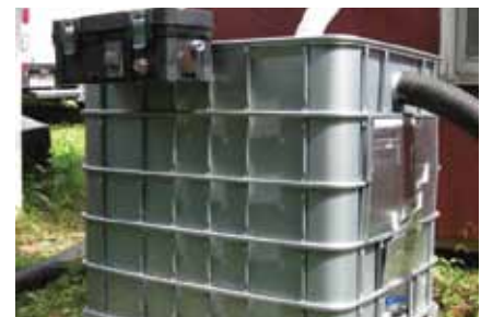
Aboveground small cistern with solar pump
