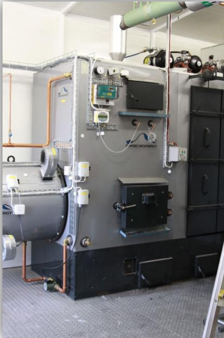
Advanced European wood combustion technology. This 500kW (1.7 MMBtu/hr) biomass boiler produces minimal particulate emissions (0.01 lbs/MMBTU) and operates with an efficiency of nearly 90%.
