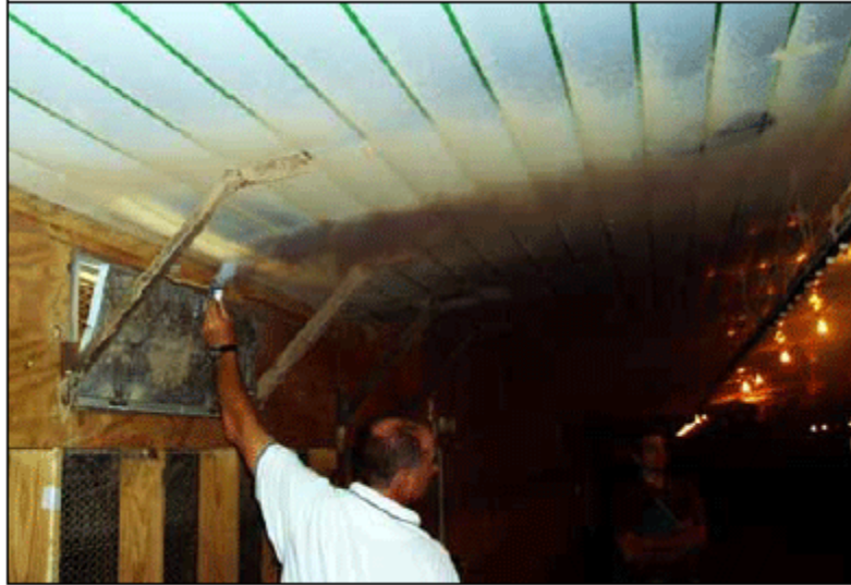
Figure 3. Air flow from a side wall inlet open two inches with a static pressure of 0.10 inches
