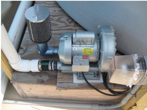
Figure 4 Blowers, pumps, tanks and heaters are important components of setting systems
