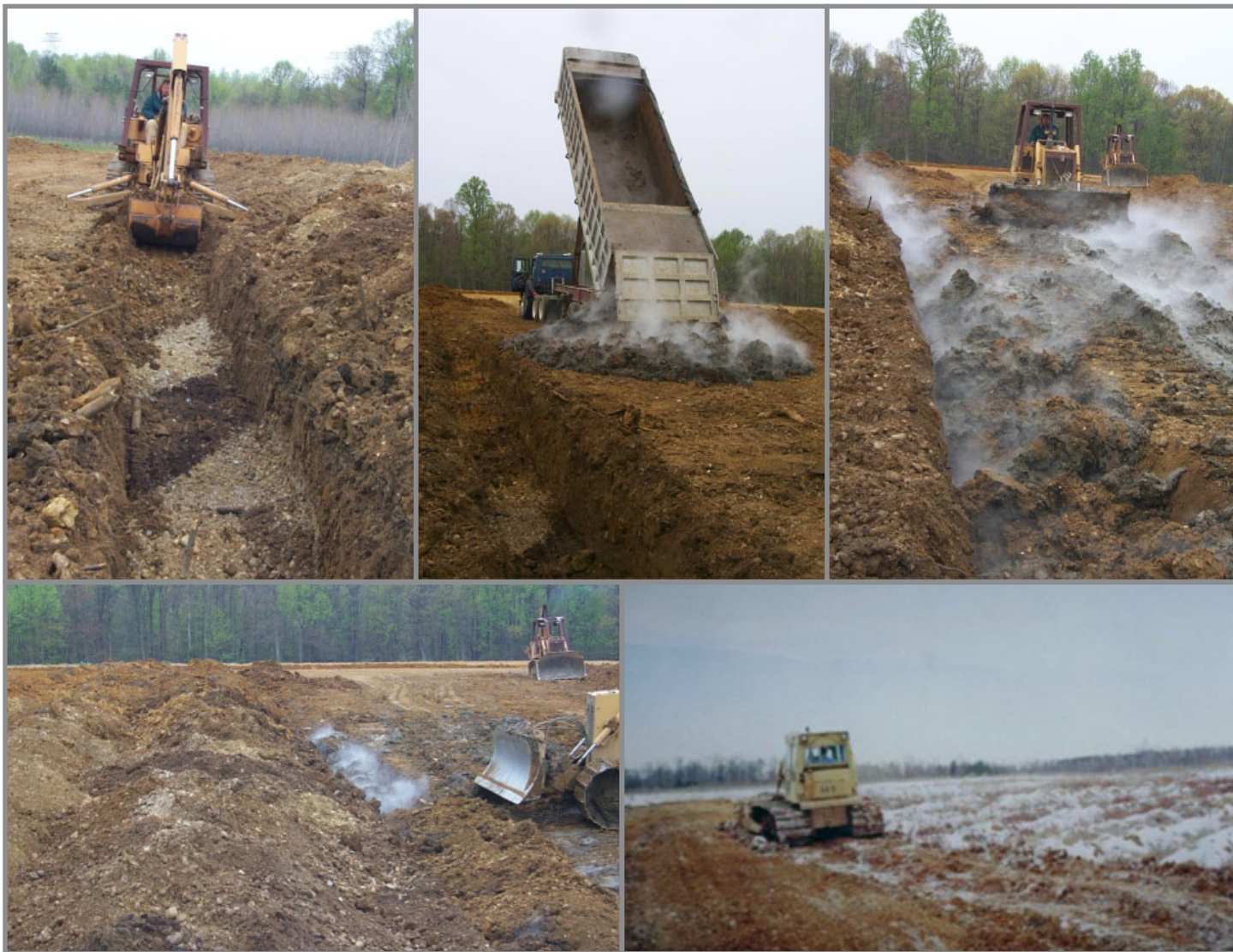
Figure 5. Pictures show progression of DRE. A trench is dug with a backhoe and biosolids deposited next to the deep row are pushed into the deep row and quickly covered. The site is graded and ready for planting.
