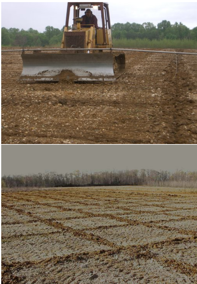
Figure 2a, 2b. a) Bulldozer with subsoiling bar and 10' boom attached. b) 10' by 10' planting grid. Hybrid poplar cuttings were planted at the grid intersections.
