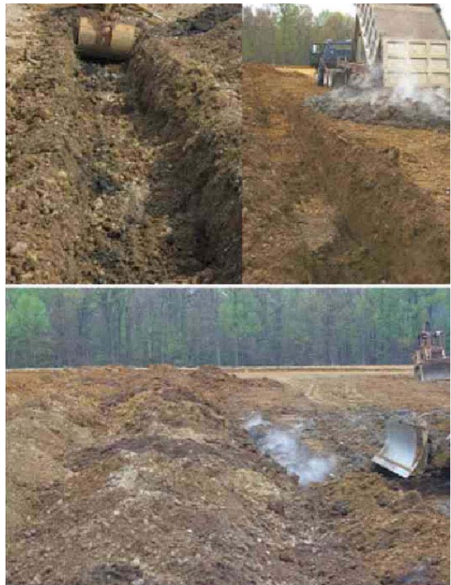
Figure 3. These pictures show the process of digging a trench, filling it with biosolids, and covering the trench with
