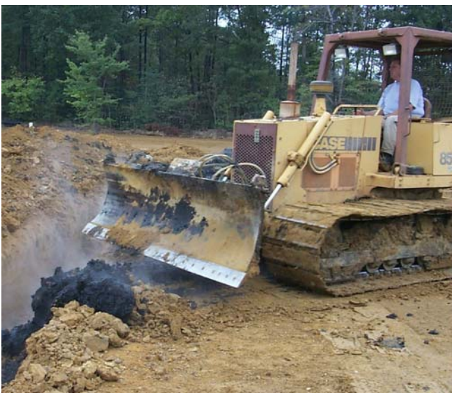
Figure 2. Bulldozer filling trench with biosolids. Greater profits result when more biosolids can be applied to an area.
