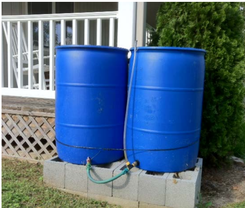
These rain barrels collect rain water from the roof of the Dorchester Historical Society in Cambridge. Photo courtesy of Dorchester Citizens for Planned Growth.
