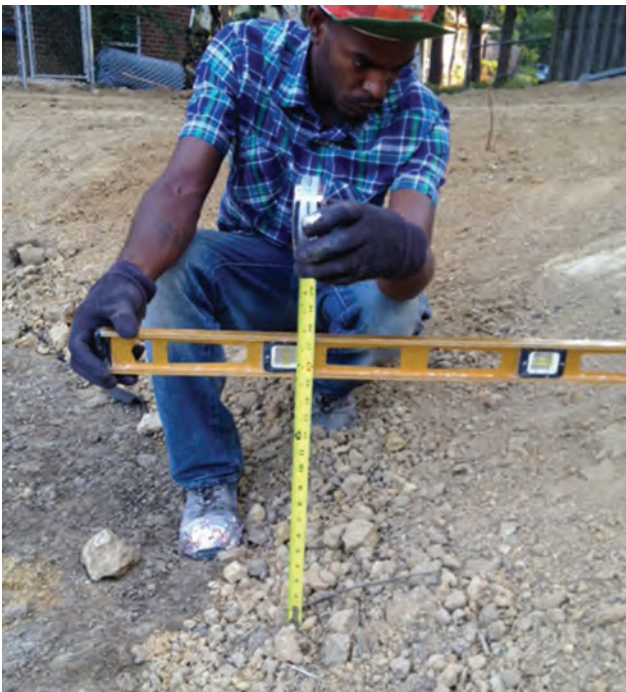
Figure 2.13. Double-check elevations throughout the construction process to ensure each layer is at the correct height according to the Rain Garden design.
